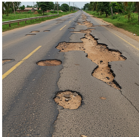
Road deterioration in ECOWAS Region
